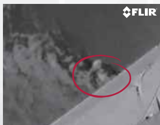
Captured gas leak from production site.
