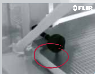
A leaking pressure gauge.
